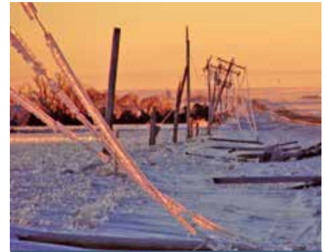
Non-VR2® cables fall to the weight of ice and force of wind. Photo taken by Ross Riley
