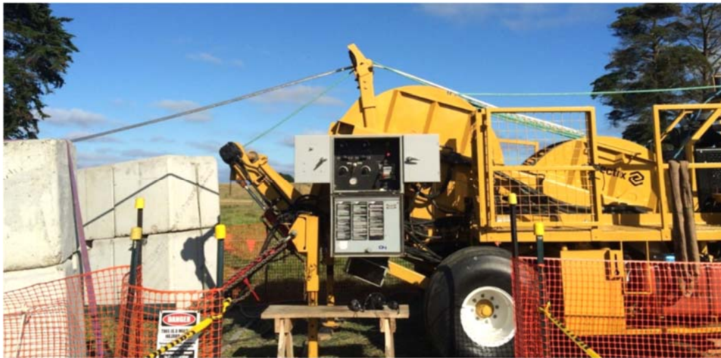
Figure 8. Adverse interaction of conductor with roller, courtesy of Transpower New Zealand.
